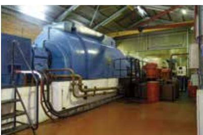
GAS TURBINE ALTERNATORS
